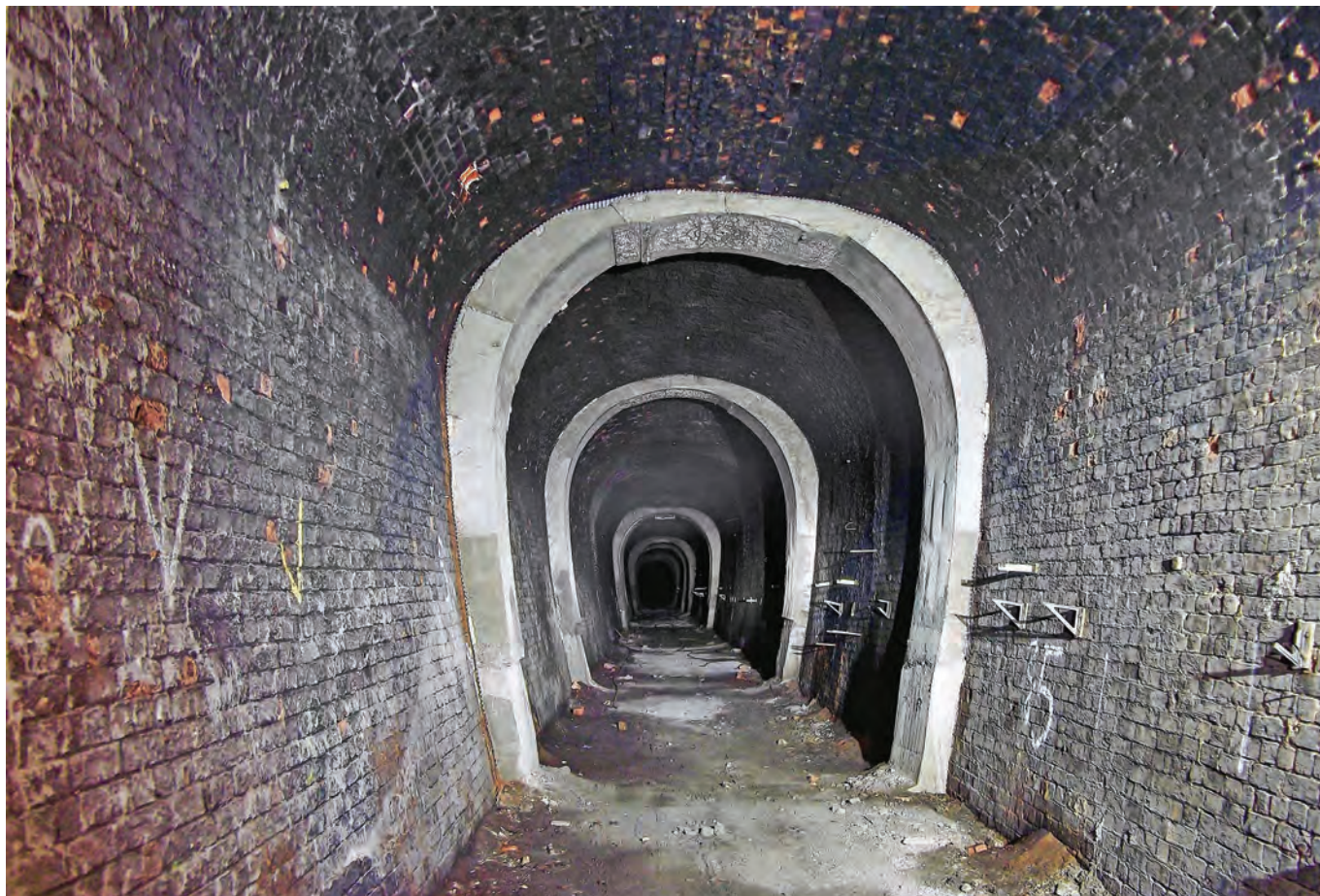
Reinforced concrete hoops used to reinforce the tunnel in places of weakness by Leicester City Council. Photo Ade Armishaw
